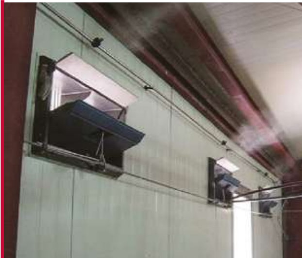
Figure 112 Example fogging system for a cross-ventilated house.
