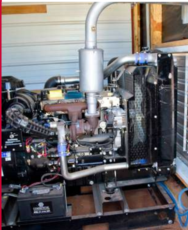
Figure 93 Example of a back-up generator.
