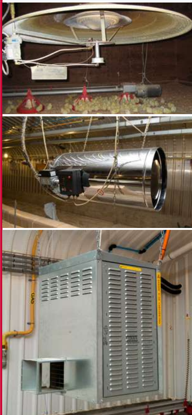
Figure 94 Examples of different house heating systems (from top to bottom, canopy brooder, whole-house heating and space heater).
