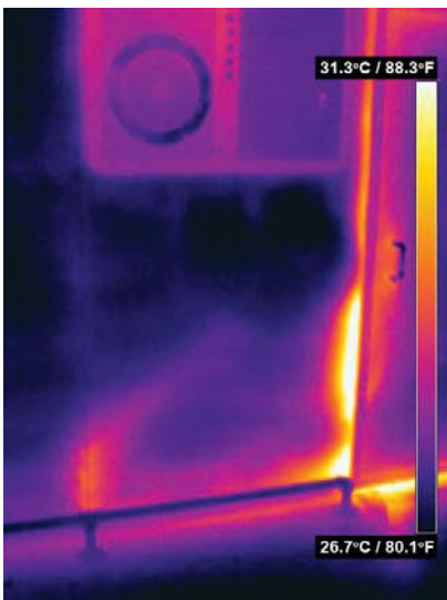
Figure 5: Thermal camera image of heat loss through poorly maintained door seal.
