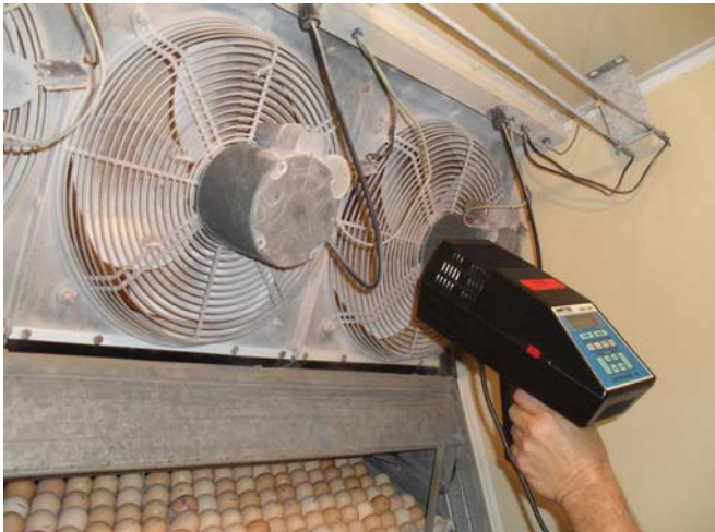
Figure 6: Using a strobe light to check fan speeds.
